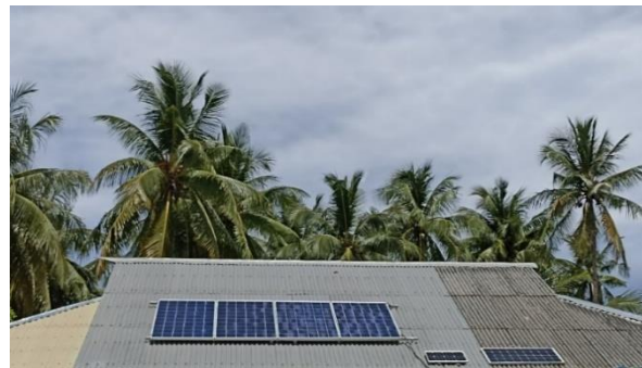
Figure 7. Solar panels installed on roofs
