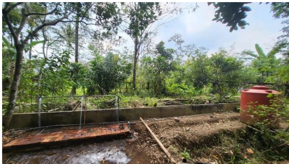
Figure 4. Water Reservoir and Faucet
