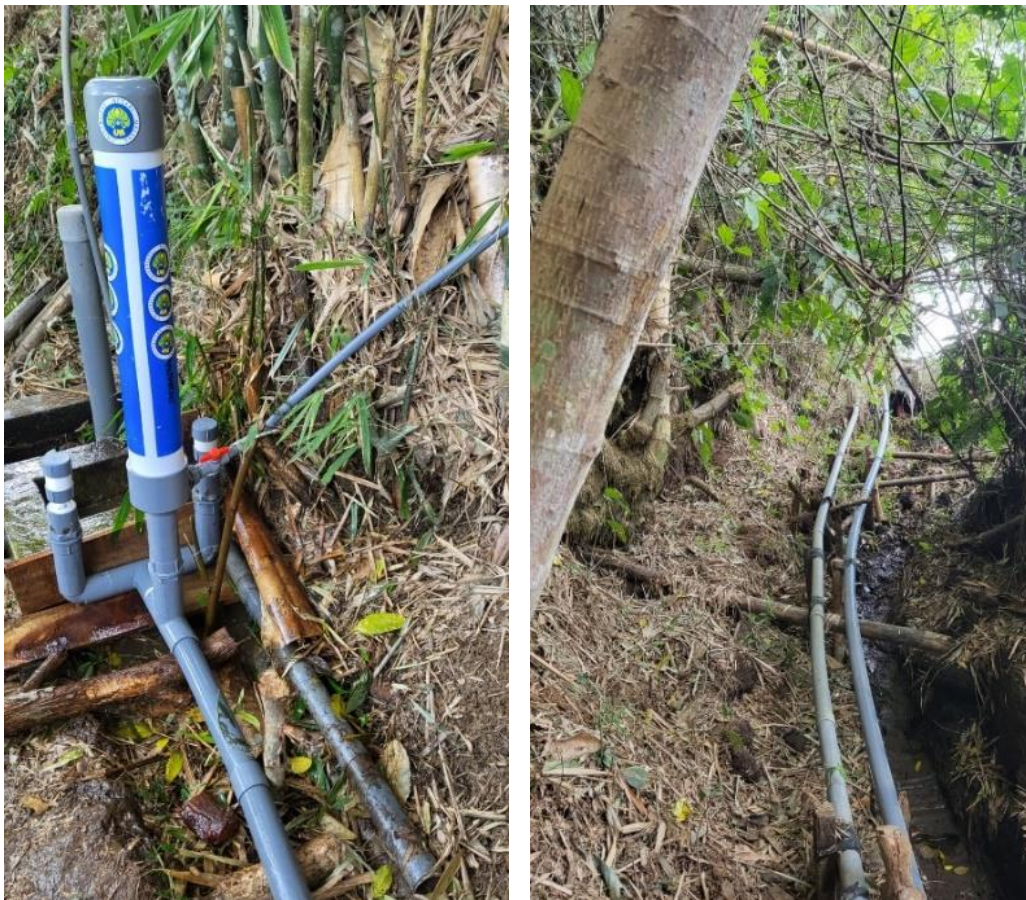
Figure 2. Non Electrical Water Pump
