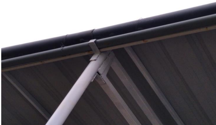
Figure 7. Small Pipes and Gutters as Water Tanks
